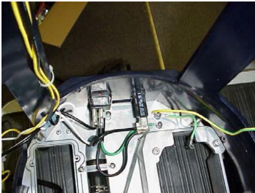
Figure 19. Power switch and circuit breaker.
