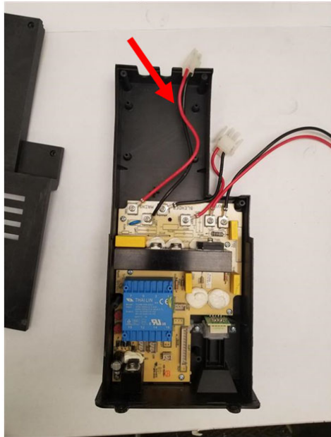
Picture of INCORRECT WIRING
